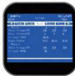
UPS Cabinet Control Panel
